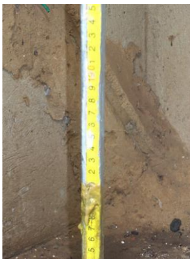
Figure 3. Depth tool with sludge markings.
